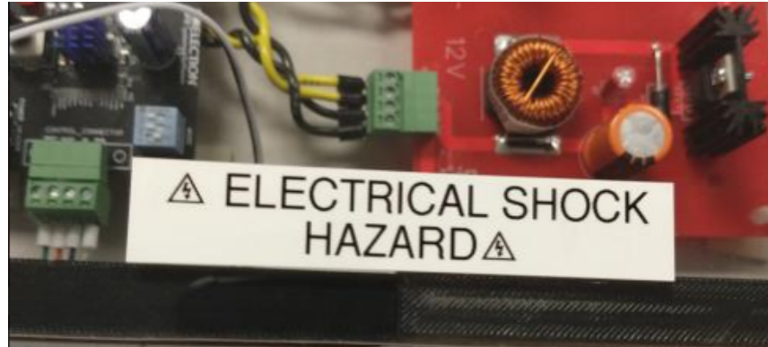
Figure 33: Electrical Shock Hazard Label
